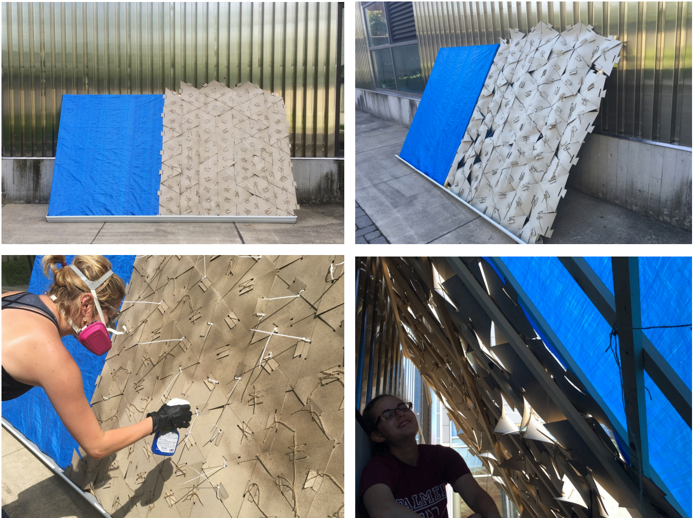
Figure 3: Paper wall process. Top right: Initial installation of tarp and paper walls. Bottom left: Hydrophobic treatment with commercially available nano-coating. Top left: After two rainstorms. Bottom right: Quality of light below the walls.
